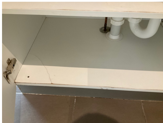
General maintenance - sink is now not leaking at the time of inspection
